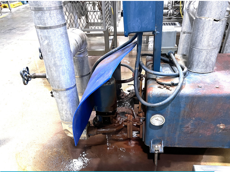
Figure 5: Electric Pump Failure: Lack of Sufficient NPSH
