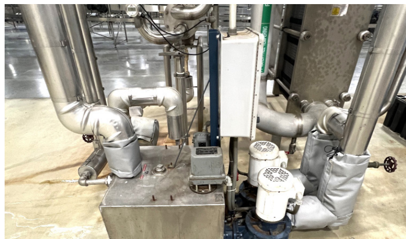
Figure 2: Condensate On/Off Pumping Unit
