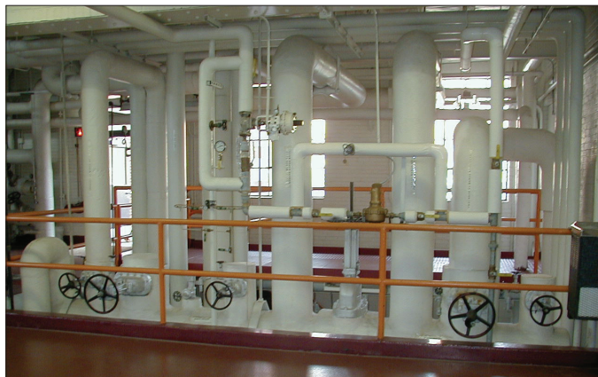
FIGURE 1. An SOP is important for properly maintaining a steam-supply system
