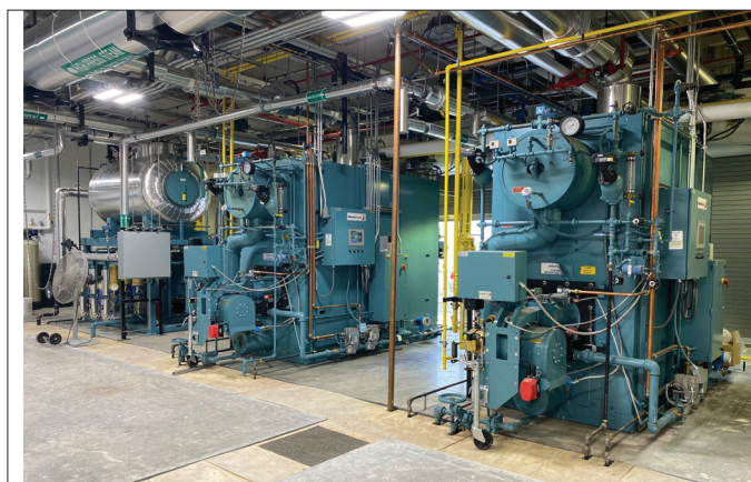
FIGURE 2. An SOP will help ensure the proper operation of a boiler plant
