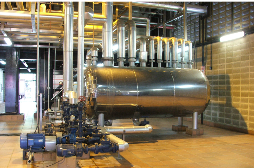
Figure 1: New Pressurized Condensate Tank System
