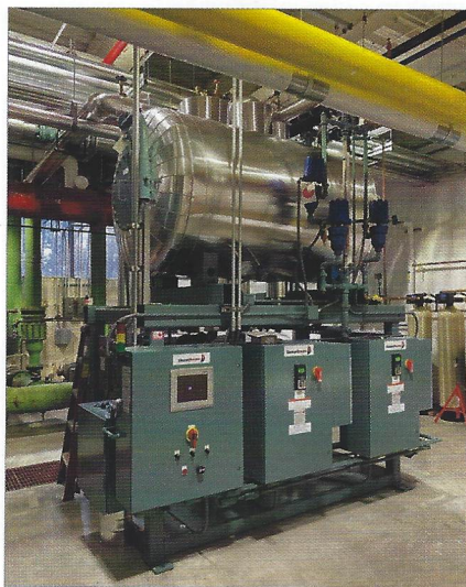
FIGURE 5: New deaerator at the BASF boiler plant. Courtesy: Inveno Engineering, LLC
