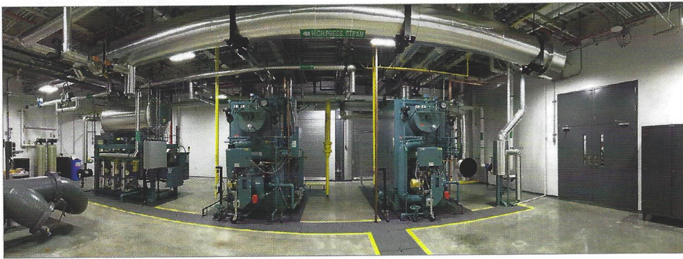
FIGURE 6: It was important to BASF to have a clean, well-organized and well-lit environment for the boiler plant personnel that provides an excellent work environment and work habits. Courtesy: Inveno Engineering, LLC
