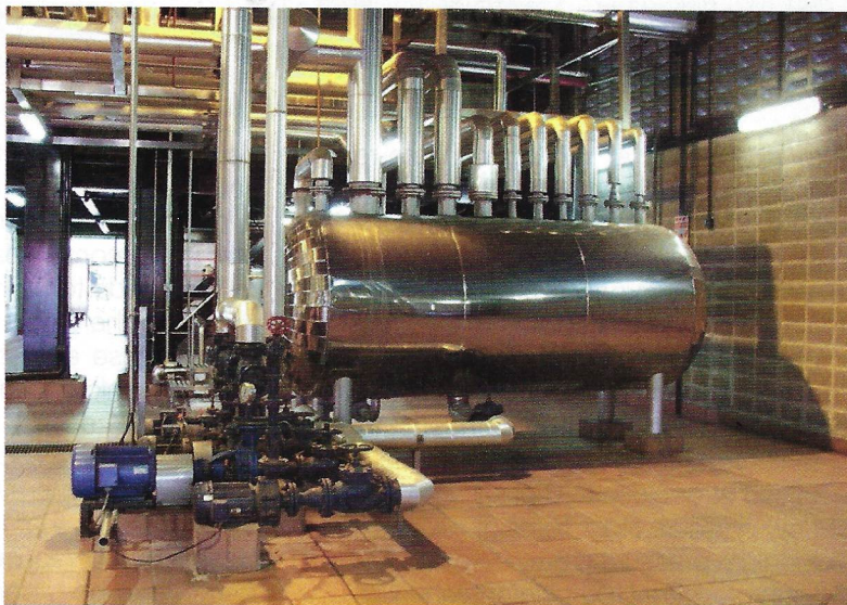
FIGURE 1. Pressurized condensate tank systems, like the one shown here, can help maximize efficiency in a plant's steam generation
