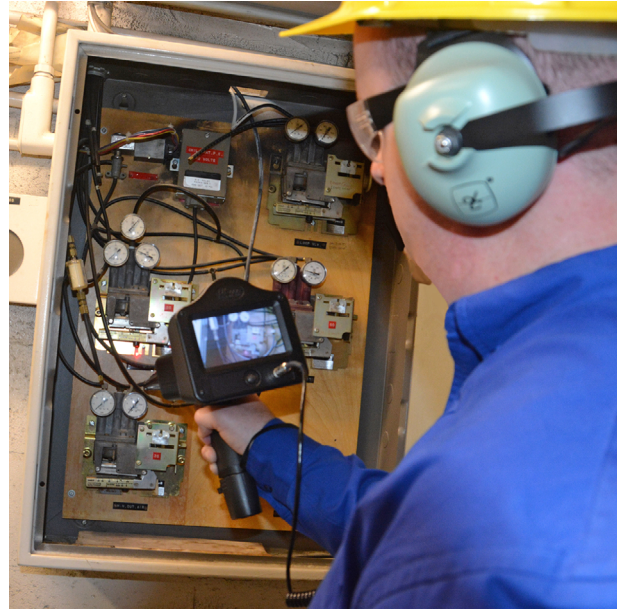
An ultrasonic detection gun is among the most effective methods of pinpointing the location and severity of compressed-air leaks.
