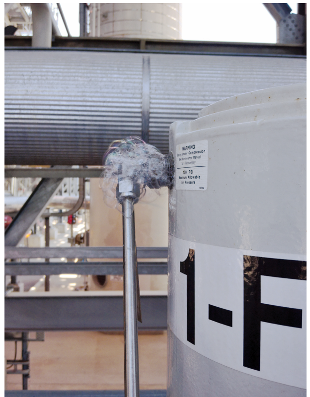
This view shows bubbles forming at a suspected leak site. The relatively large size of the bubbles indicates a substantial leak at low pressure.
