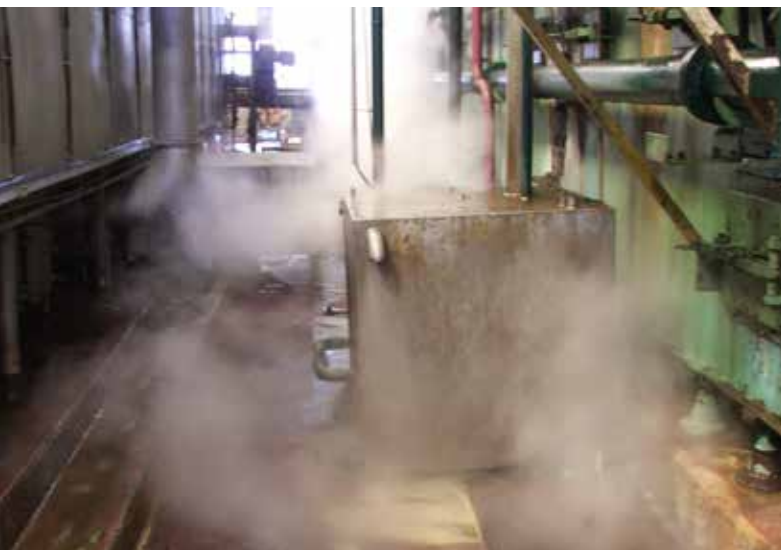
Figure 1: Electric Condensate Pump Failure
