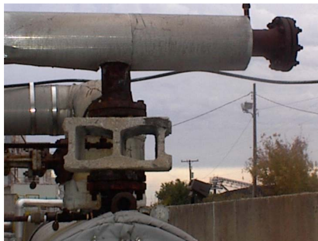
Figure 24. Piping Not to Code
