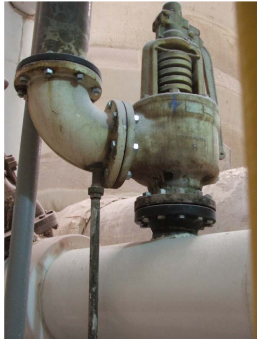
Figure 20. Discharge Vent Line Attached to the Safety Valve: Installation Is Incorrect
