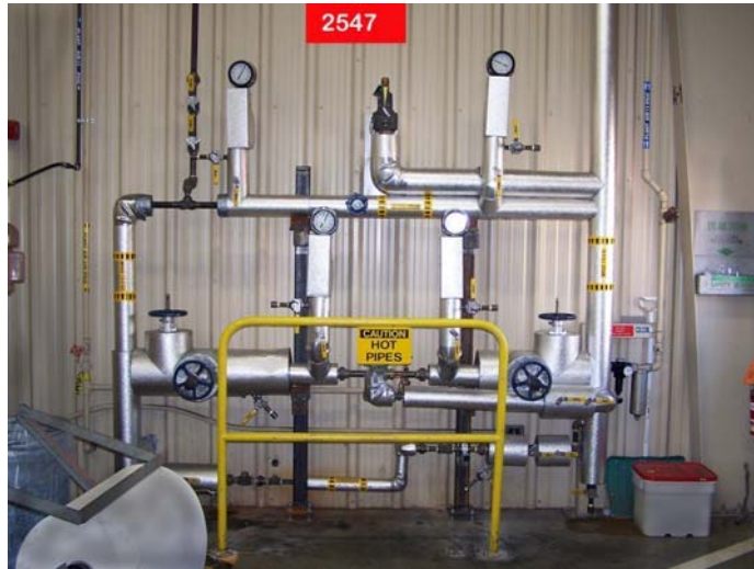
Fig. 1. Newly constructed steam pressure-reducing station.
