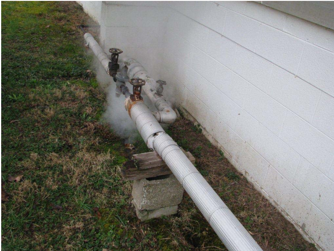
Fig. 2. Leaking steam piping and deficient piping support.
